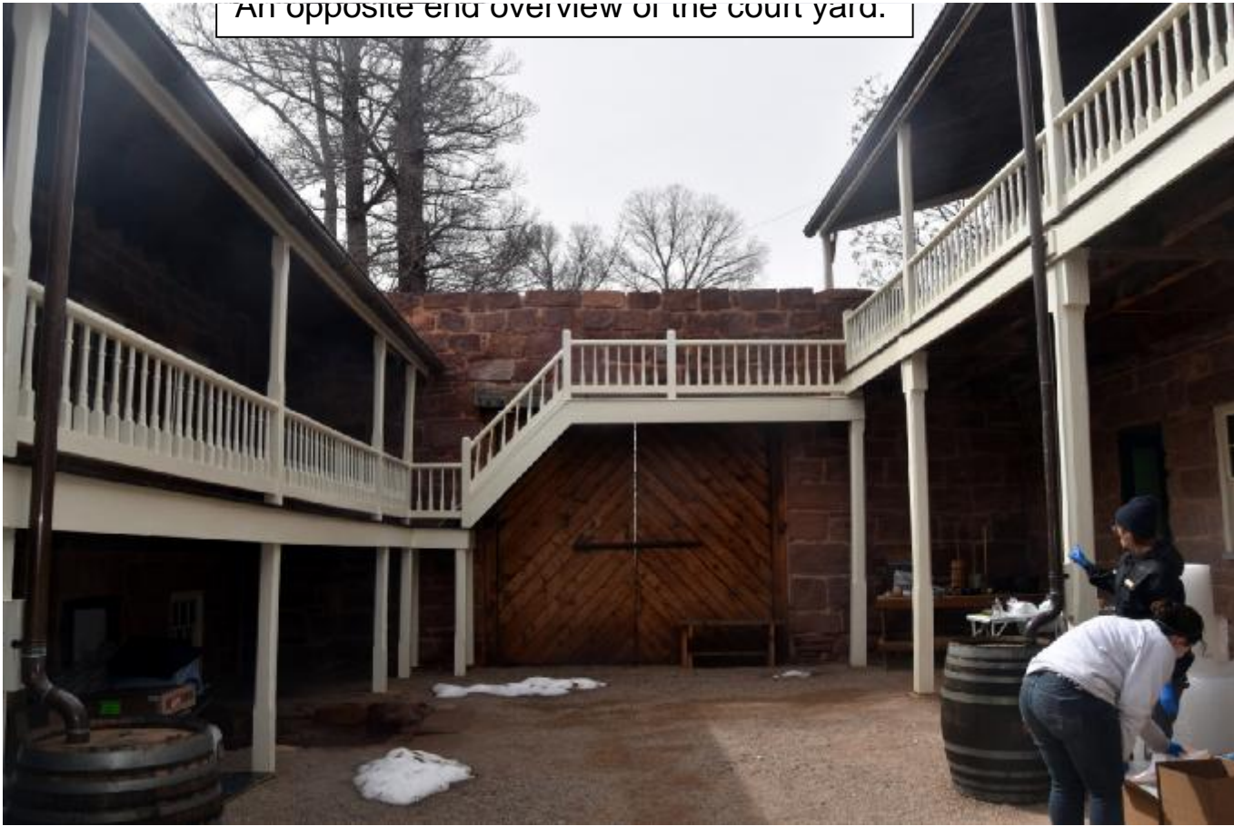
An opposite end overview of the court yard.
