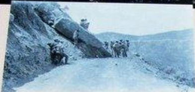
Much like today, work crews in the 1930s were kept busy clearing the park road. — Photo courtesy of Denver Public Library — Western History Department
