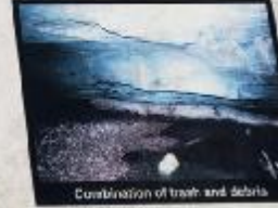
Combination of trash and debris
